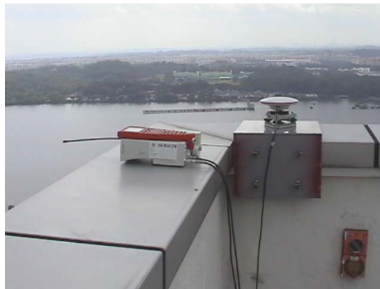
Figure 4: The monitoring station, R1
