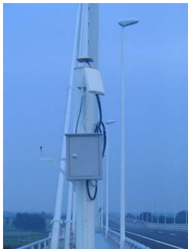
Figure 6: GPS sensor mounted on the bridge deck
