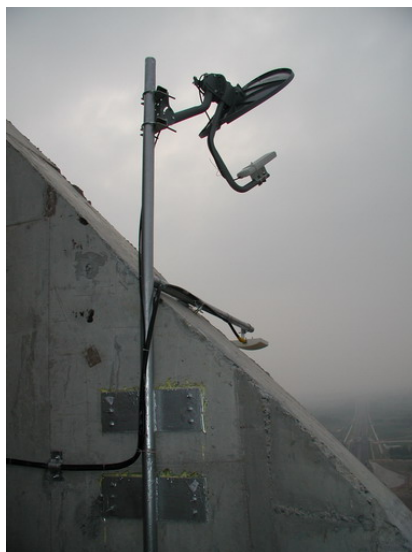
Figure 11 Wireless bridge at the top of the bridge tower
