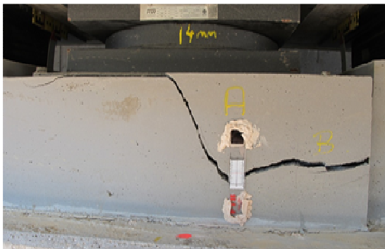
Figure 3: Crack in the bridge After these activities it was decided to use a long-term, permanent monitoring system for the further observation.
