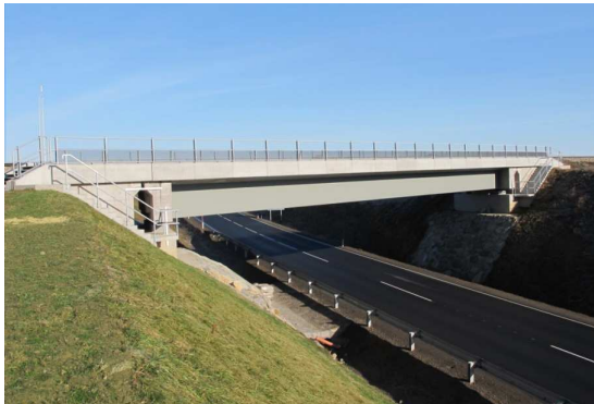
Figure 2: OBB-Bridge Großhaslau (Lower Austria) During the construction progress in 2010 cracks have been observed, which led to surveys from summer to spring 2010. The bridge became monitored in behalf of the ÖBB Infrastructure company (Krems) and the settling could be stopped by structural engineering methods.
