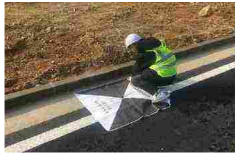
② Air photo signal
