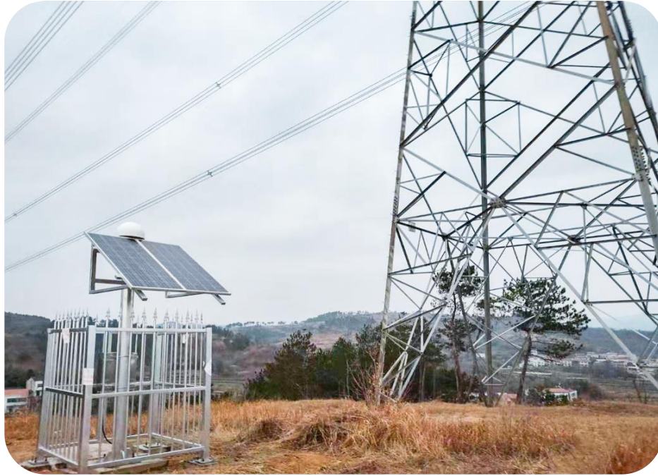
GNSS Monitoring for Electricity Infrastructure
